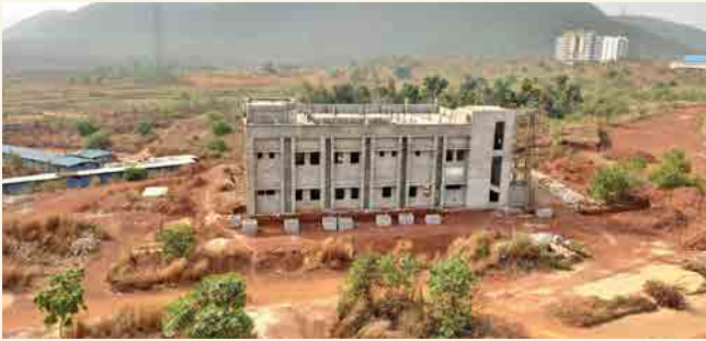
Dispensary: Structural work completed and finishing work is in progress. About 58% building work completed.
