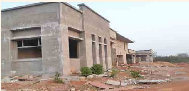
CRIF: Structural work completed and finishing work is in progress. About 81% of building work completed.
