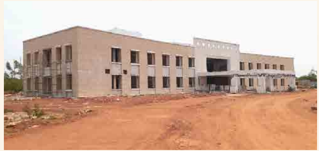
SHSSM: Structural work completed and finishing work is in progress. About 93 % of building work completed.
