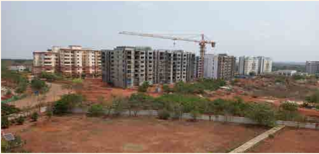
Type-C1 & C2 Quarters: Structural work completed and finishing work is in progress.
