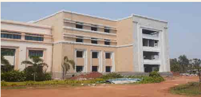
SIF Extension: Structural work completed and finishing work is in progress. About 69% of building work completed.
