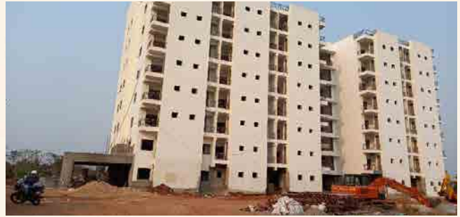
Efficiency Hostel: Structural work completed and finishing work is in progress. About 73% of building work completed.
