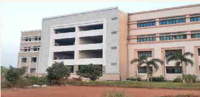
SBS Extension: Structural work completed and finishing work is in progress. About 69% of building work completed.
