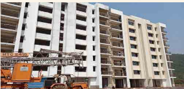
Type-D1 & D2 Quarters: Structural work completed and finishing work is in progress.
