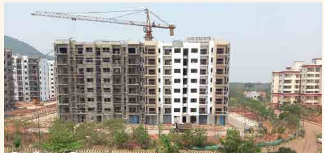
Type-B3 & B4 Quarters: Structural work completed and finishing work is in progress.
