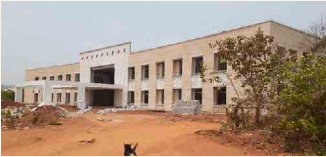
SEOCS: Structural work completed and finishing work is in progress. About 93% of building work completed.
