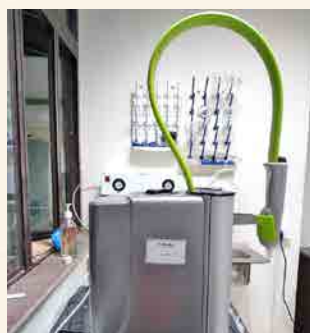
A newly installed water deionization unit in the Molecular Biology laboratory of SKBET
