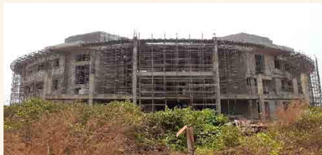
LHC-1: Structural work completed, Dome work and other finishing is in progress. About 77% of building work completed
