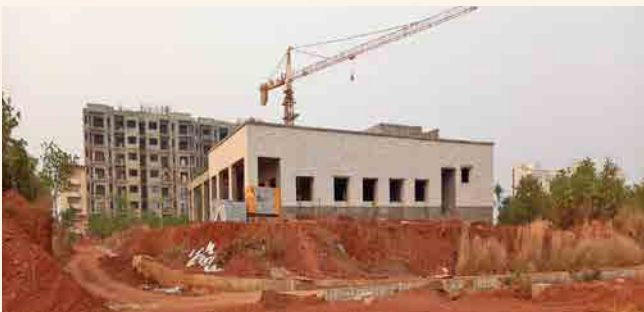
Commercial Complex (Residential): Structural work completed and finishing work is in progress. About 42% of building work completed
