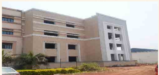
SMS Extension: Structural work completed and finishing work is in progress. About 69% of building work completed.
