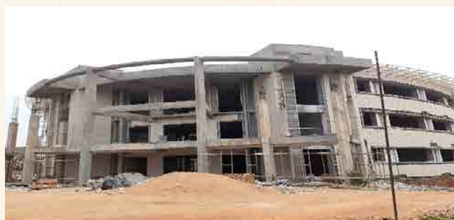
LHC-3: Structural work completed and finishing work is in progress. About 93% of building work completed.
