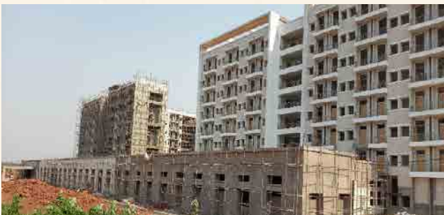
Boys' Hostel-3: Structural work about 72% completed and finishing work is in progress
