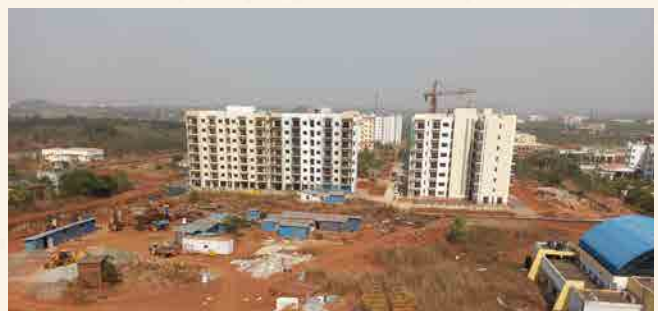
Type-A1 & A2 Quarters: Structural work completed and finishing work is in progress.
