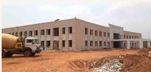
SMMME: Structural work completed and finishing work is in progress. About 93% of building work completed.
