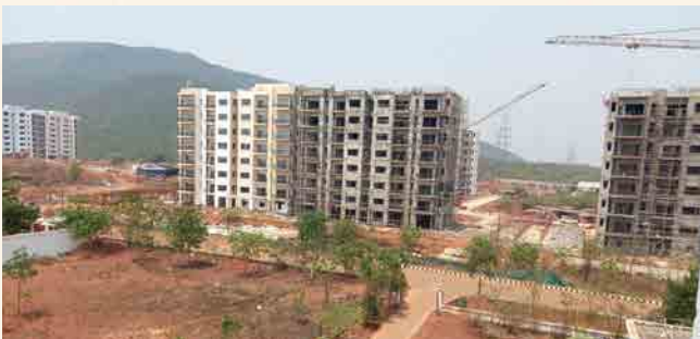
Type-B1 & B2 Quarters: Structural work completed and finishing work is in progress.
