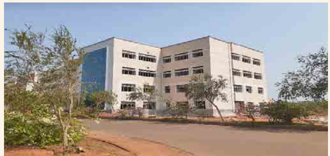
SES Extension: Structural work completed and finishing work is in progress. About 84% of building work completed.
