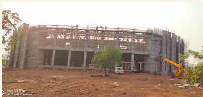
Auditorium: RCC structural work completed, roof truss work & other finishing work is in progress. About 57% of building work completed
