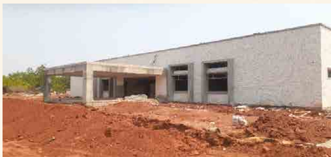
Central Workshop: Structural work completed and finishing work is in progress. About 82% of building work completed.
