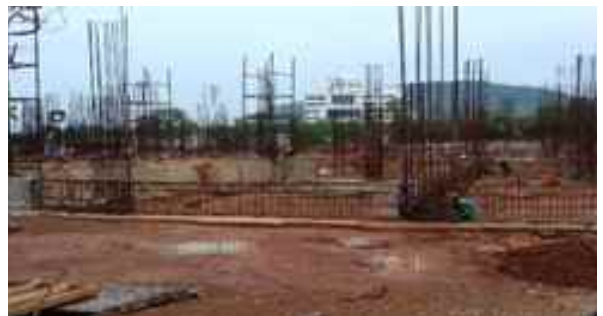
LTC-1: Plinth beam and column work above plinth beam are in progress.
