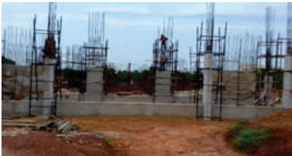
LTC-3: Plinth beam and column work above plinth beam are in progress.
