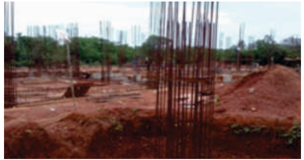
HSSM : Plinth beam work and column above plinth beam works is in progress.
