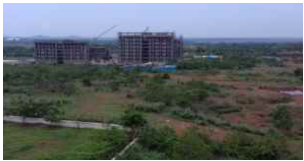
Boys' Hostel-2: A wing terrace completed. 7th floor block work is in progress. B wing fifth floor column work is in progress and 3rd floor block work is in progress.
