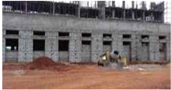
Boys' Hostel-2: B wing 3rd floor roof slab casted. Column work is in progress. 2nd floor block work is in progress and front side block work completed.
