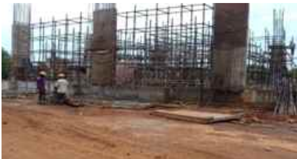
LTC-2: Plinth beam and column work above plinth beam are in progress.
