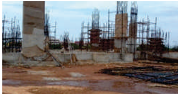
LTC-2: Plinth beam and column work above plinth beam are in progress.
