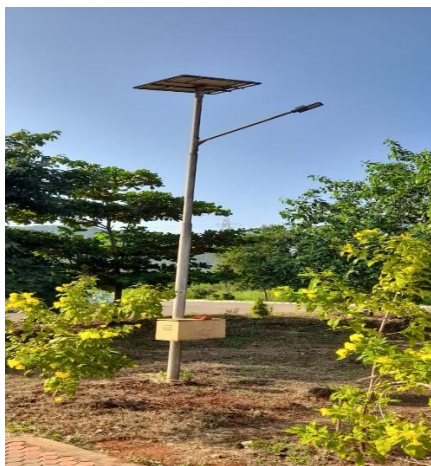
Solar Street lights.
